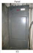
(C) Panel - This electrical device contains either multiple breakers or fuses and is used to distribute power to multiple locations within a building and/or unit.
